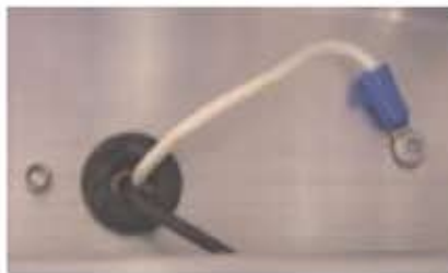
Lights are independently grounded.
